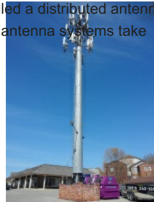
A monopole planted in the back of a shopping center.
