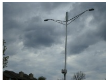
Street light cell site above a major thoroughfare.
